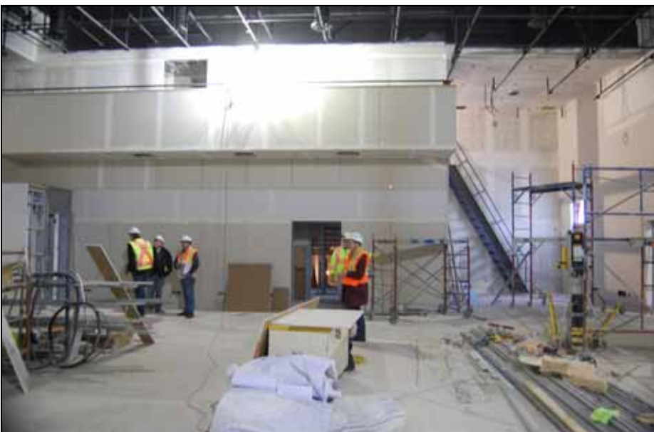
Looking stage left to right onstage of the Conklin. The stairs lead to a storage area above the green room and booth & gallery access.
